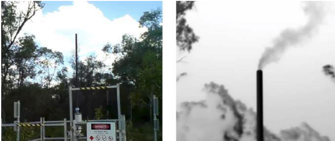
Figure 0-3: Methane emissions from gas-well de-watering pipeline (Source: Tim Forcey)
