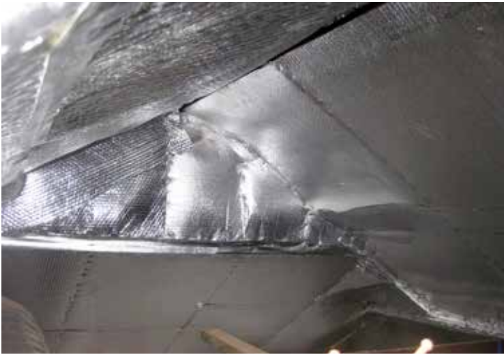
← Aircell Retrosshield was stapled to the underside of the roof as part of the roof space insulation.
