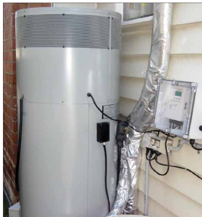
Heat-pump storage hot water unit showing the solar controller at the right-hand-side and insulated pipes to the collector.
