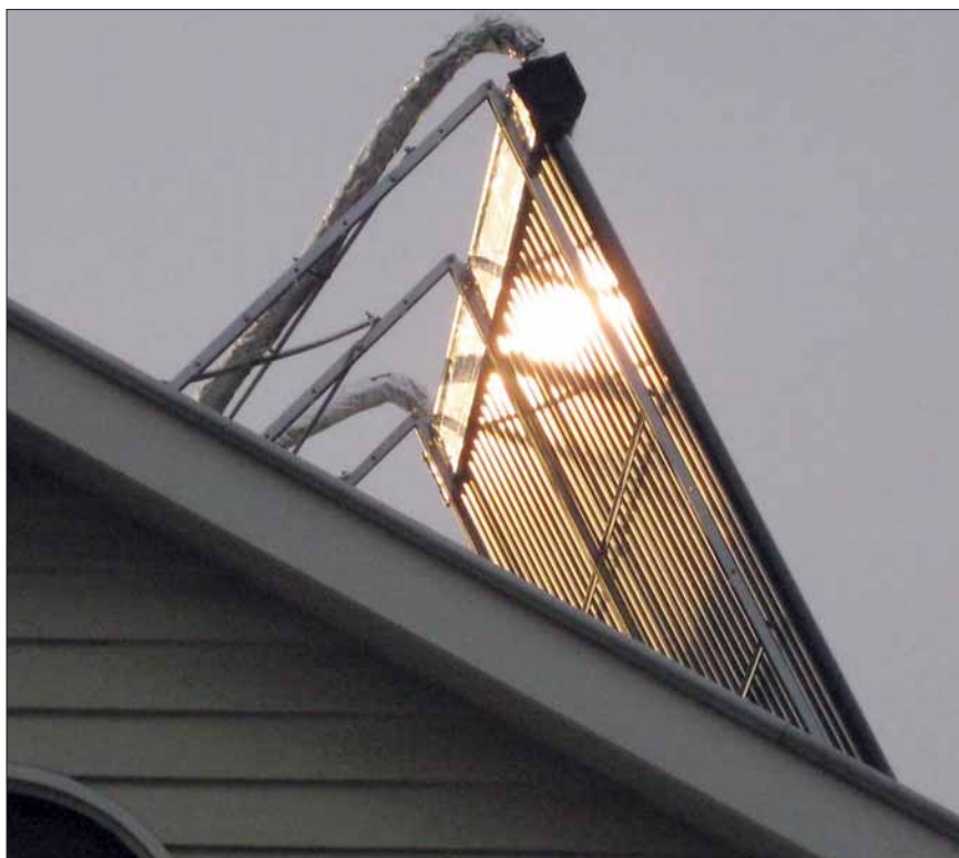
The solar collector tilted at 64°. In summer the early morning and late afternoon sun actually heats the evacuated tubes from behind!
